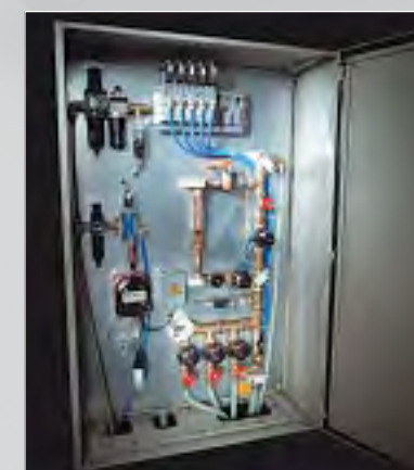
Pneumatic and process water distribution
