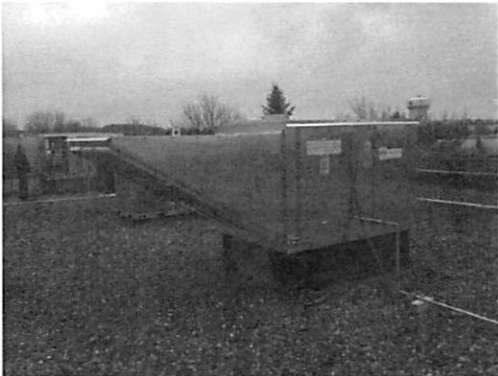
Horizontal outdoor down discharge (Roof-mounted)
